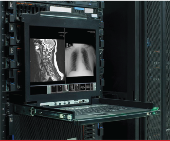
IT and Server Rooms
